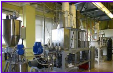
The co-generation power plant (CEM-10)
